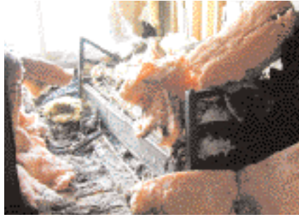
Life safety is an obvious motivator for homeowners considering RFS systems.
