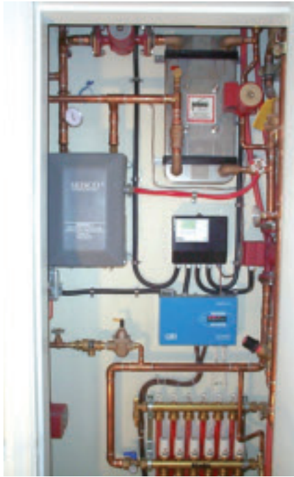
Closet space housing the mechanical system was 10" deep by 30" wide in PNE home.
